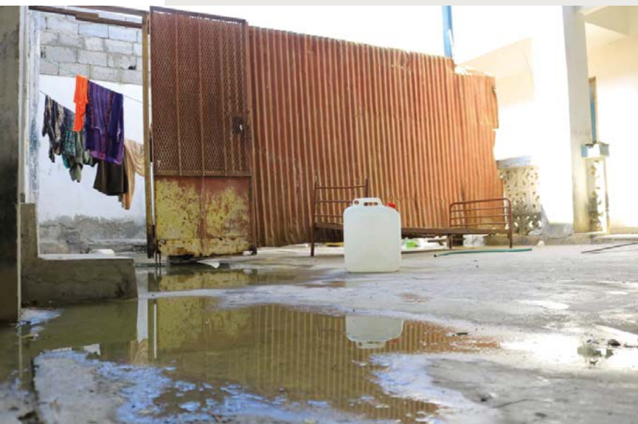
The Al-Hudaydah central prison, in Yemen, before support was provided to improve the conditions of women inmates. © OHCHR
